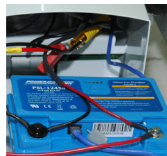
Fig. E (Battery terminals) Located in back on Ascend EL
